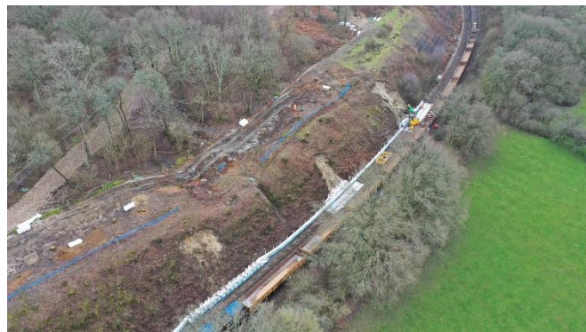
An aerial view of the landslips near High Brooms. Credit: Network Rail
